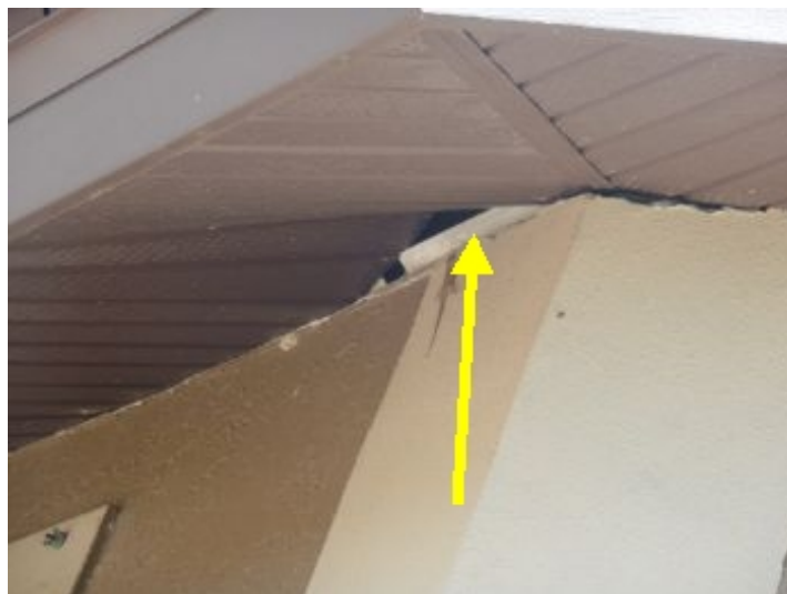
Soffit dented at front right of home
