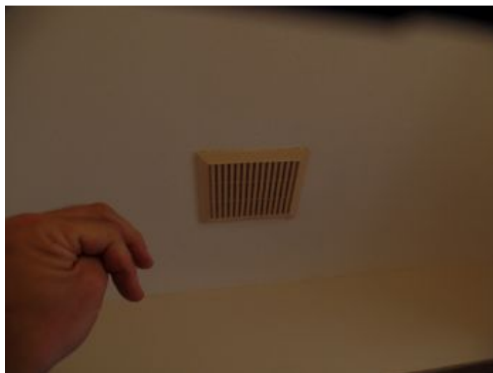
Unit is very noisy at the upper guest bathroom
