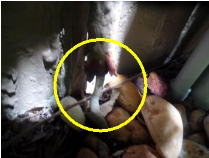
Unprotected wiring at rear right of home
