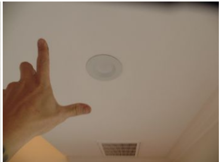
The front entry light fixture did not respond to the control. This could be a burnt/ missing bulb or a dead circuit
