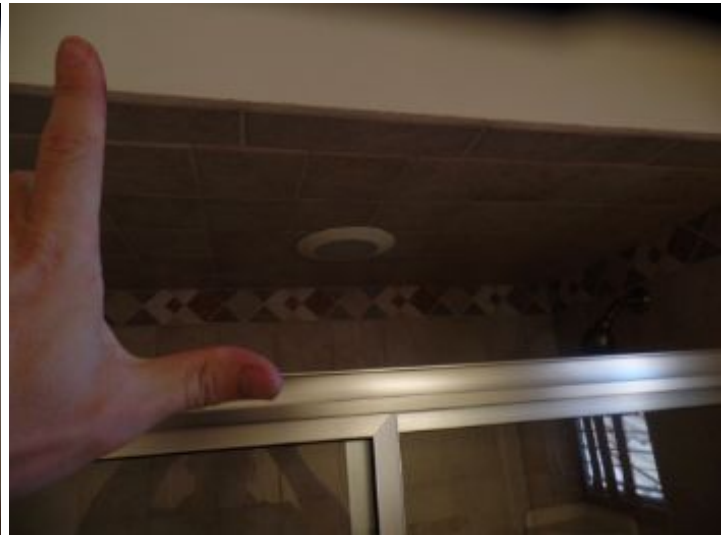
The guest bath ceiling light fixture did not respond to the control. This could be a burnt/ missing bulb or a dead circuit
