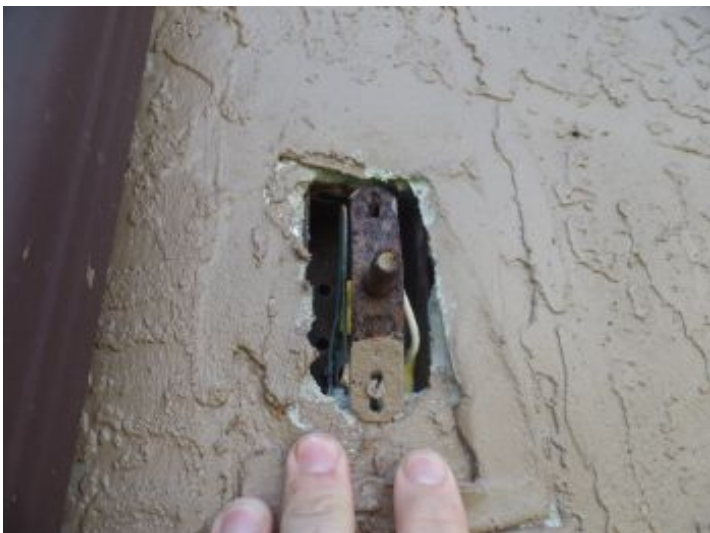
Open box at rear left exterior wall ( missing fixture )
