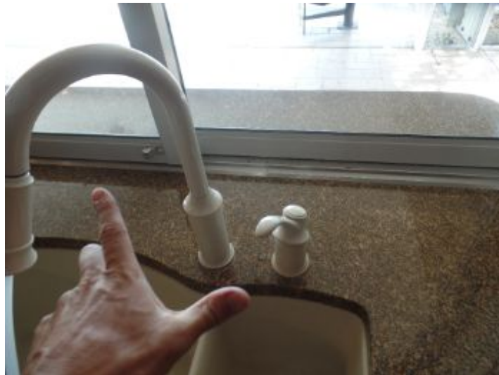
Kitchen faucet and handle were loose to counter top. Handle was worn
