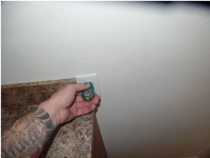
There is no GFCI (Ground Fault Circuit Interrupter) protection for all recommended electrical outlets in the utility room or right side exterior
