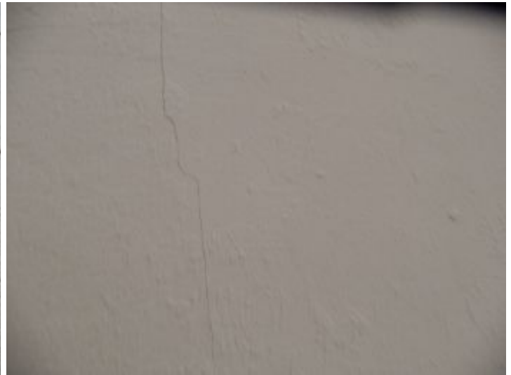
Minor cracks (1/8" or less) present in interior walls. Generally speaking, cracks that are less than 1/8" are not commonly regarded as being structurally significant. Nonetheless, they should be monitored to see if there is active movement in this area.
