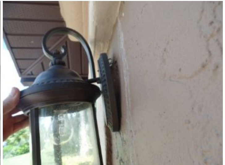
Recommend sealing light fixtures at garage front walls to the stucco wall to help prevent water intrusion
