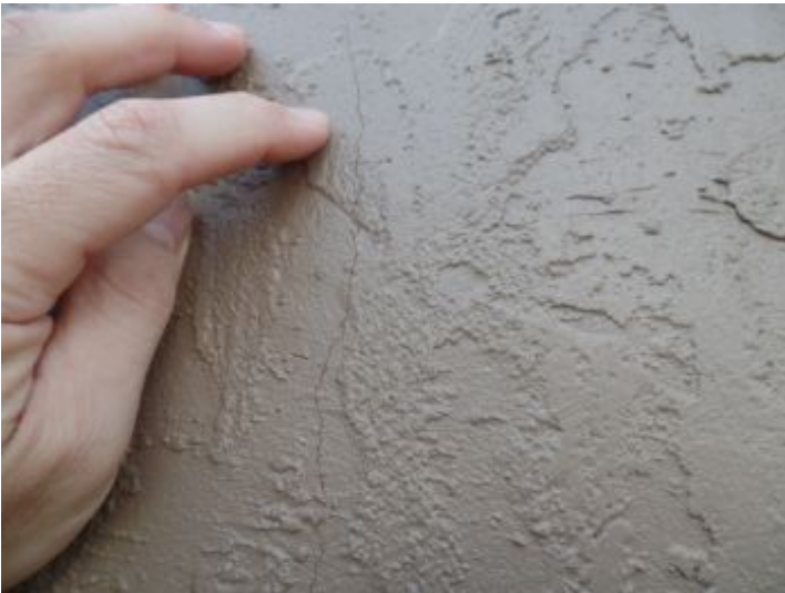
Minor cracks / holes (1/8" or less) present in exterior wall. Consider sealing them to prevent water infiltration. Generally speaking, cracks that are less than 1/8" are not commonly regarded as being structurally significant. Nonetheless, they should be monitored to see if there is active movement in this area.
