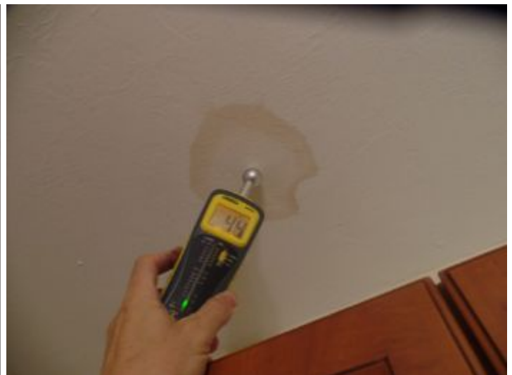
Stain visible at butler pantry ceiling, This was tested with a moisture meter and found to be non active at this time, however we recommend monitoring
