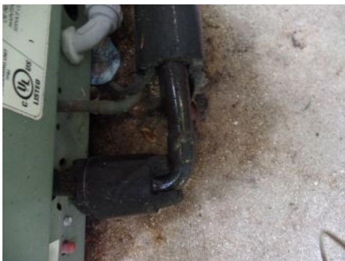
Refrigerant lines insulation is deteriorating at the outside units
