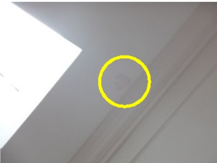
Small stain visible at living room near the sky light. Could not test due to ceiling height
