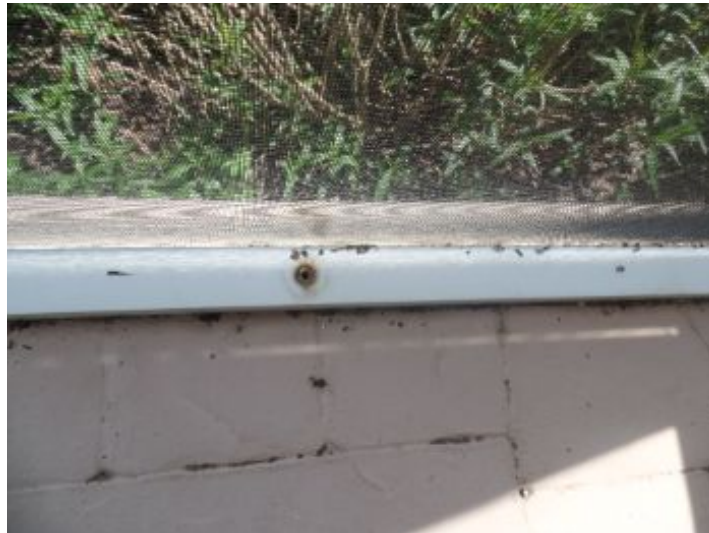
Fasteners are rusting and missing at various areas on the screen cage, mainly at the bottom track deck connection
