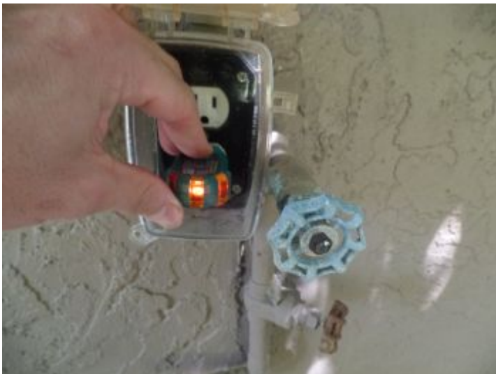
There is no GFCI (Ground Fault Circuit Interrupter) protection for all recommended electrical outlets in the utility room or right side exterior
