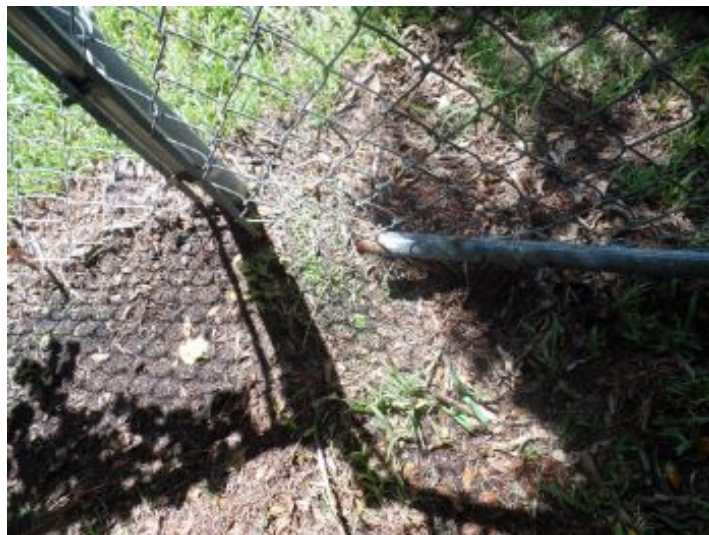
Fence damaged at front right of home
